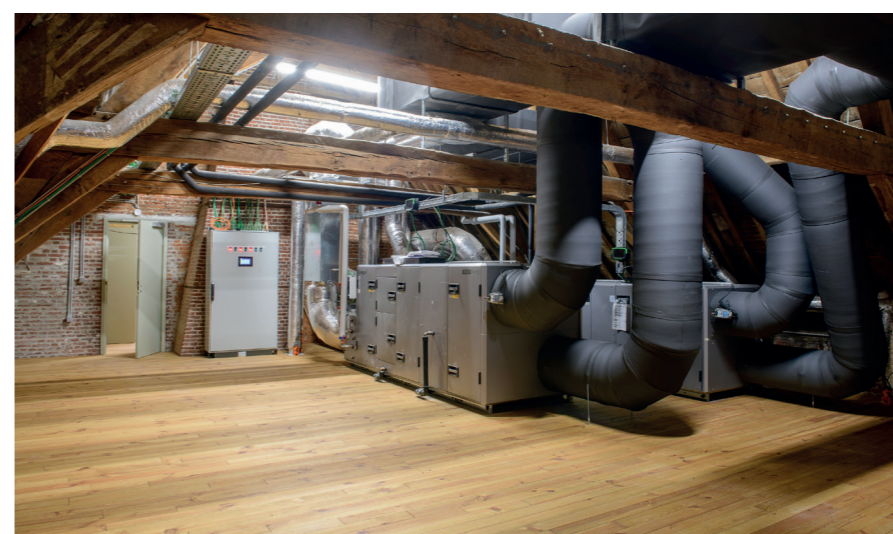
Technical installation in the attic. © Jo Exelmans
