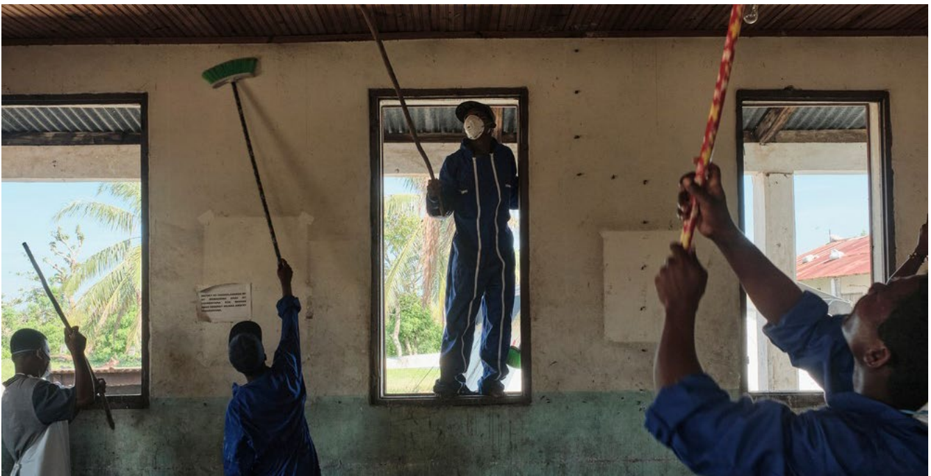
[MSB122807] Construction workers rehabilitate the hospital in Nosy Varika, Madagascar, after it was damaged by cyclones Batsirai and Emnati in February 2022. The storms were the latest in a series of shocks the country has faced in recent years. 1,2 iAko M. Randrianarivelo, March 2022.
