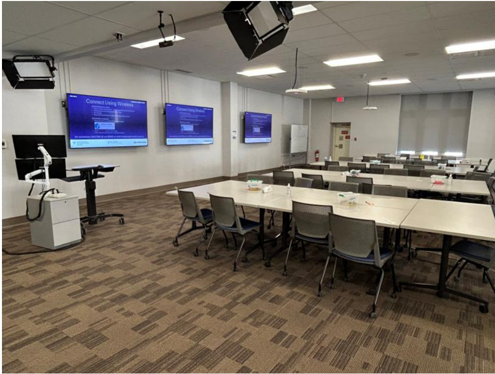
The IMS classroom utilizes advanced video technology for hybrid classes with high production values. The TCC M microphones in IMS space are used for conferencing, recording, and reinforcement using TruVoicelift simultaneously.
