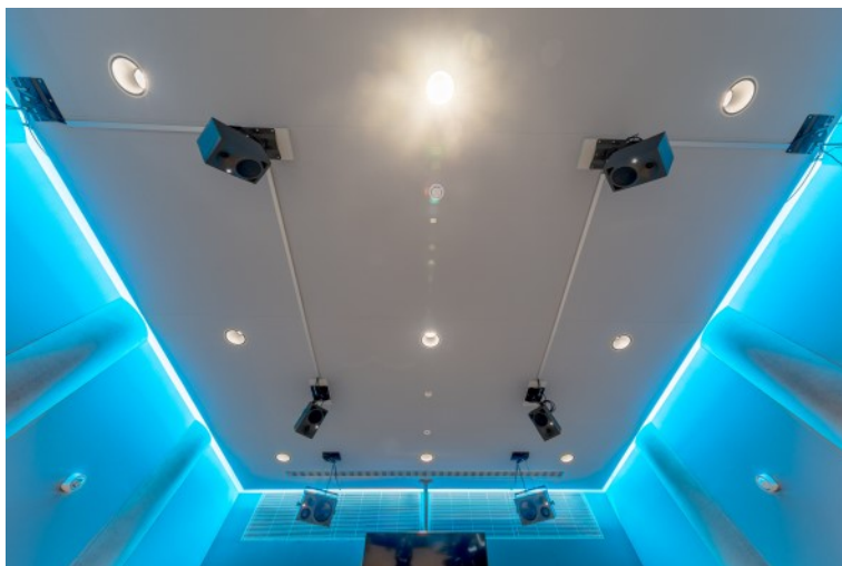
The ceiling of the 3D control room: on the elevated loudspeaker level, the inner loudspeaker circuit consists of four Neumann KH 120 for the reproduction of Dolby Atmos
