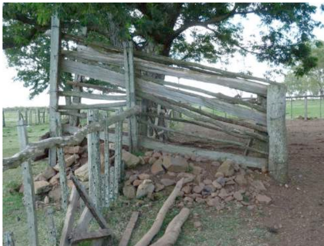
The loading ramp looks very dilapidated.
